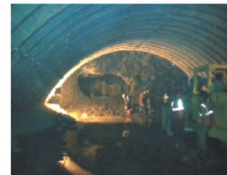
Butterfly Valve Chamber of THDC PSP project, Tehri
