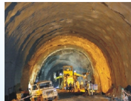
A view of Chenani - Nashri highway tunnel project under construction in J&K, NHAI
